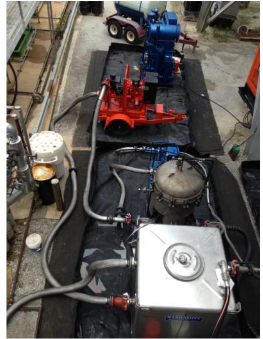
Process Equipment Setup
