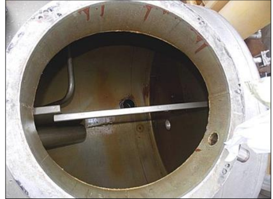
Reservoir Before Cleaning
