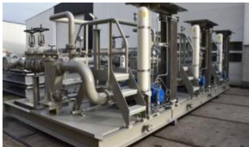
Crude oil pumps
