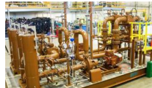
Fuel forwarding pumps
